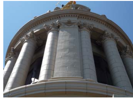
Terminal Tower, 48th and 49th floor fiberglass dentil cornice and Corinthian columns replacing terra cotta.
