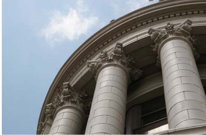
Terminal Tower, 49th floor fiberglass dentil cornice and corinthian columns replacing terra cotta.
