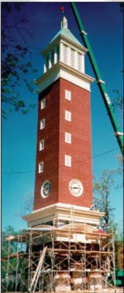
Historical Reproduced FRP Bell Tower Housing Cellular Antenna
